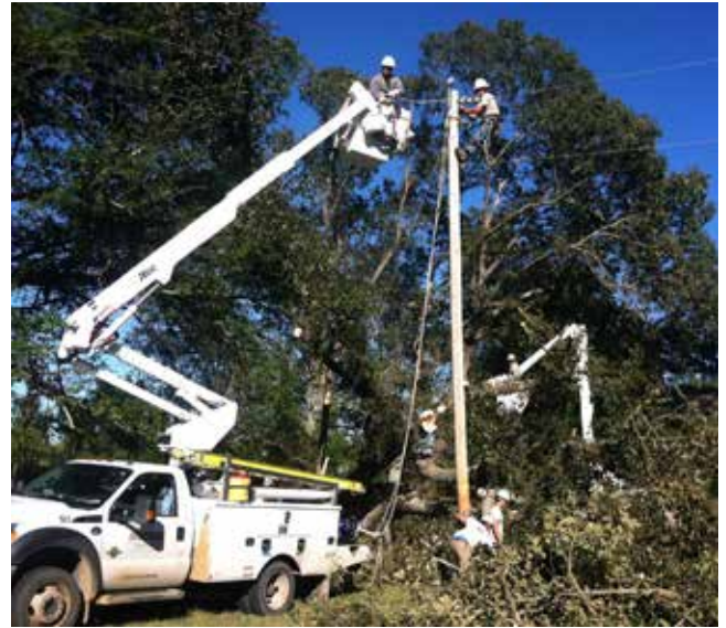
Nolin RECC line techs work to restore power in Aiken, South Carolina, where Hurricane Matthew ripped through the area leaving 9,000 members in the dark.
