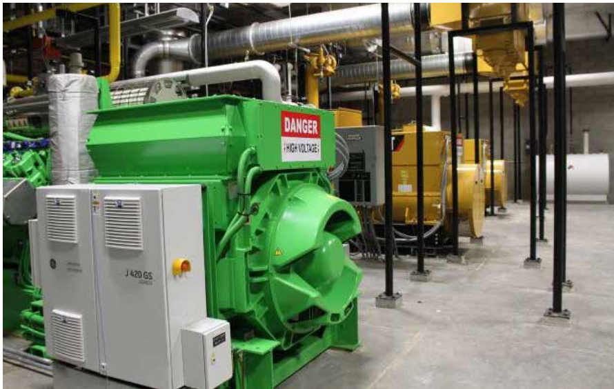
Pictured are three of Fort Knox’s natural gas generators. Photo: Dustin Ward
