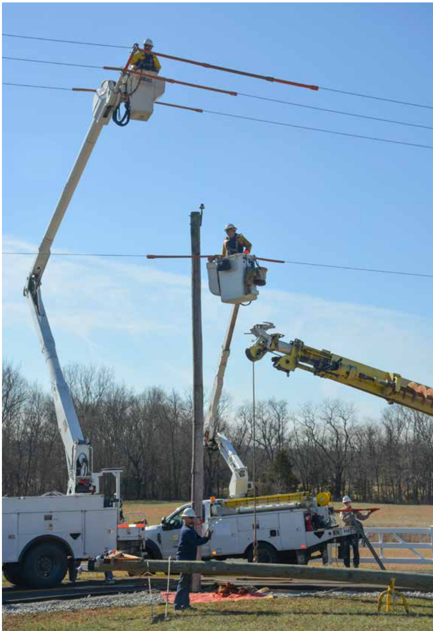
Senior Line Technician Chad Pence, top; Senior Line Technician Anthony Huff, second from top; Apprentice Line Technician Ryan Ray, bottom middle; and Crew Leader Kenny Brown change out a pole in Howe Valley.
