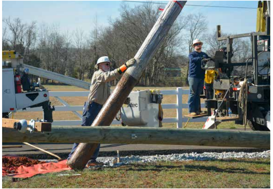
Apprentice Line Technician Ryan Ray, right, and Crew Leader Kenny Brown remove an old pole that needs replacing.
