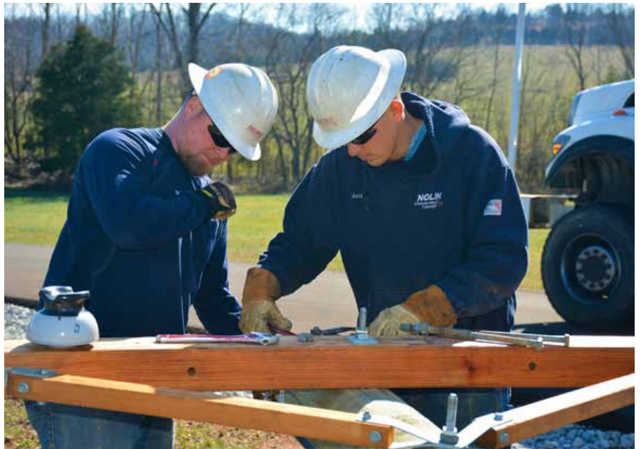
Apprentice Line Technician Ryan Ray, left, and Senior Line Technician Anthony Huff prepare a new pole for service.
