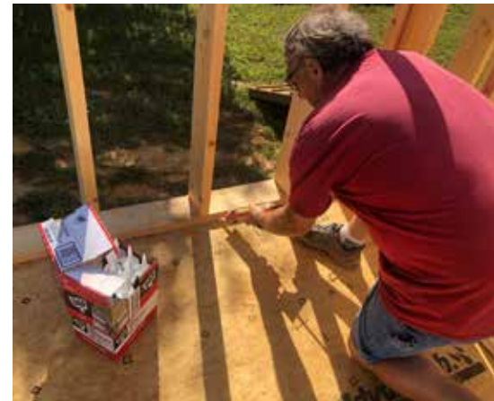
Habitat for Humanity was able to put caulk Nolin donated to good use on local homes.
