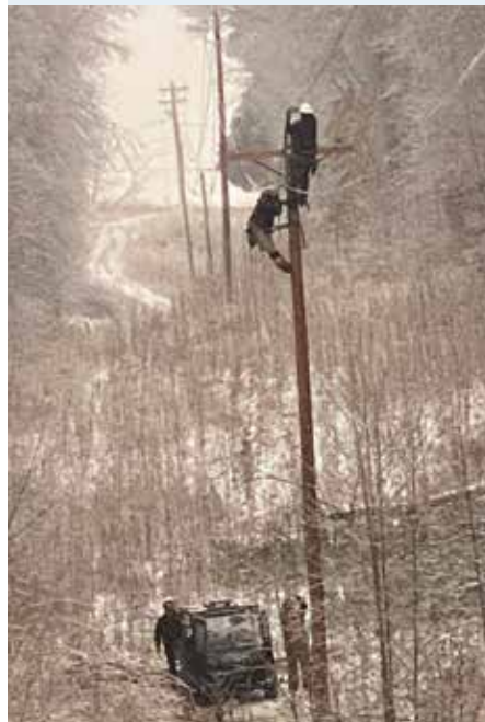
Nolin line techs work in challenging conditions at Grayson in Carter County. Photo: Nolin RECC Senior Service Technician Jamie Price
