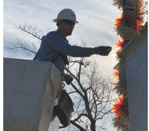
Nolin line crews were busy in November and December helping our communities decorate for the holiday season. Pictured is Nolin Line Technician Brandon Hurd putting finishing touches on the arch that welcomed residents to Christmas in the Park at Freeman Lake in Elizabethtown. Photo: Sarah Fellows
